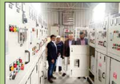
CATS- MIST (EECE) team`s factory visit in Basic Power Engg Ltd at Tongi, to inspect and test LT /HT Panel and Load Break Switch (LBS) of 11 /0.415 KV Sub-station of Mirpur Cantonment
