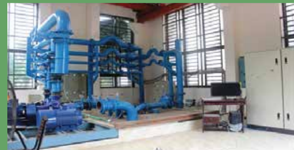
Figure 8: Pump test bench
