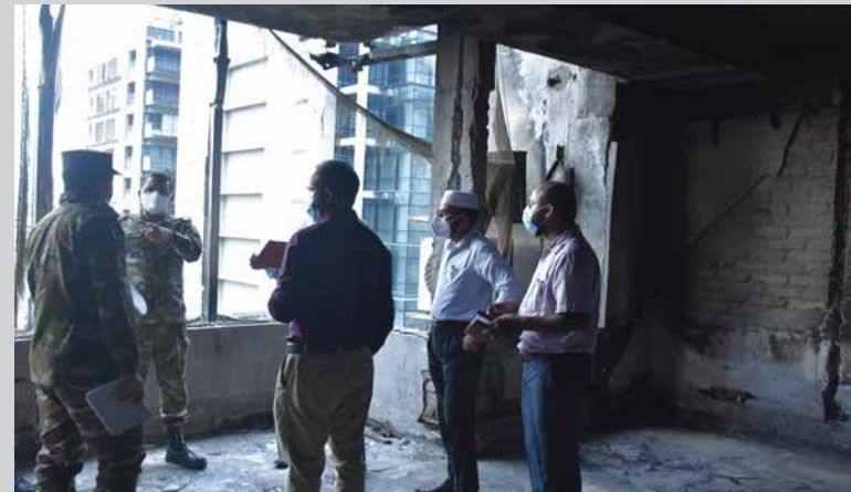
Figure 4: Post-fire damage assessment of 7 th , 8 th & 9 th floor of FR Tower, Banani, Dhaka
