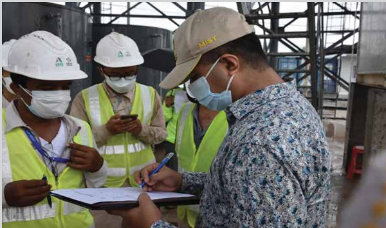
Figure 3: Batching plant calibration for Dhaka Elevated Expressway PPP Project Tranche 2 & 3 at Tejaon Plant, Dhaka
