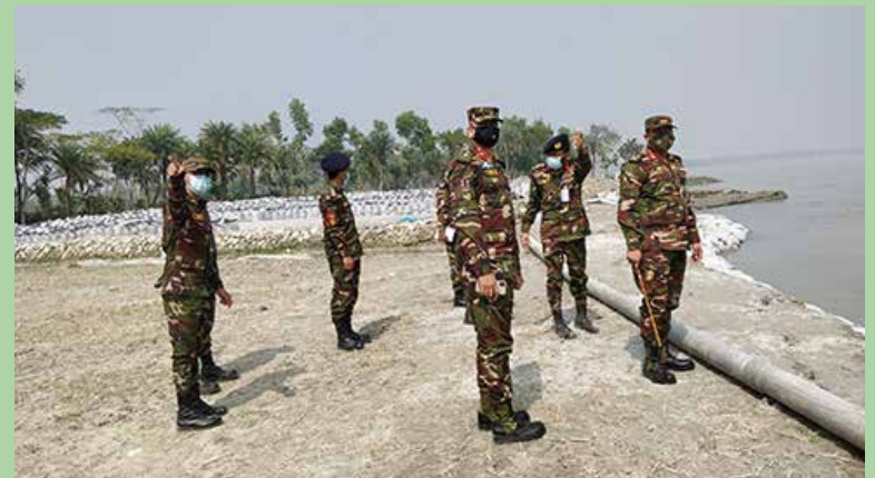
GOC 7 Infantry Division visits to the bank protection work of Sheikh Hasina Cantonment on 06 February 2021 accompanied by Director of CATS-MIST (EWCE)
